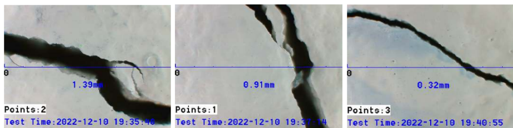
Figure 4. Photo of the scanned width of the crack
